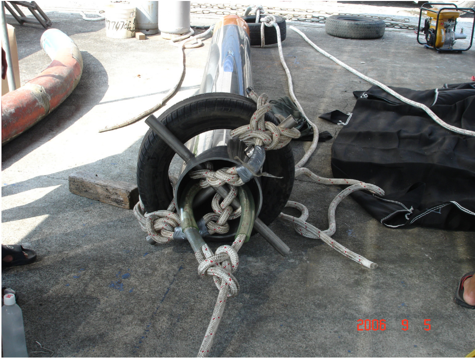
Photo A A semi-closed pipe prepared for installation (準備安裝的半封閉圓管)
